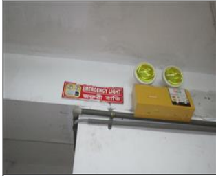
Photo of fire safety equipment Fog light.JPG
