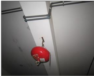
Photo of fire safety equipment Auto DCP.JPG
