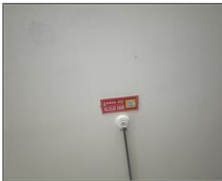
Photo of fire safety equipment Smoke detector.JPG
