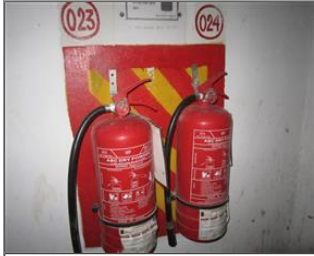
Photo of fire safety equipment Fire extinguishers.JPG
