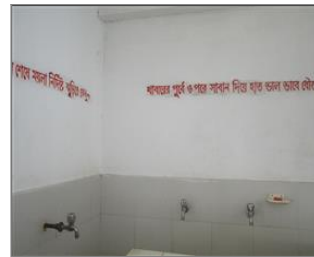
Photo of the sanitary facilities Hand wash point.JPG
