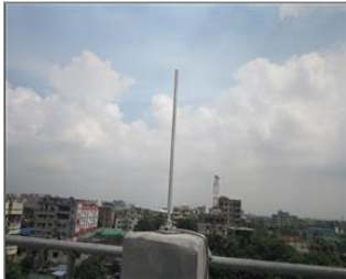
External photo(s) of the production unit(s) Lightning arrester.JPG
