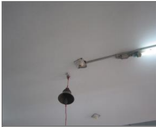
Photo of fire safety equipment Gong bell.JPG
